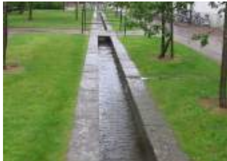
Storm Water Drains Inside the Layout
