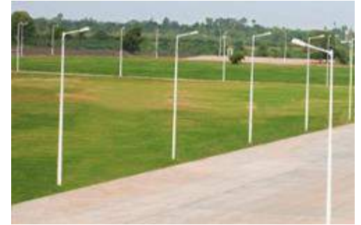
Street Lighting Inside the Layout
